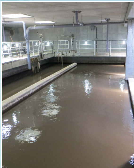
Inside the Douglas L. Smith Middle Basin Plant
