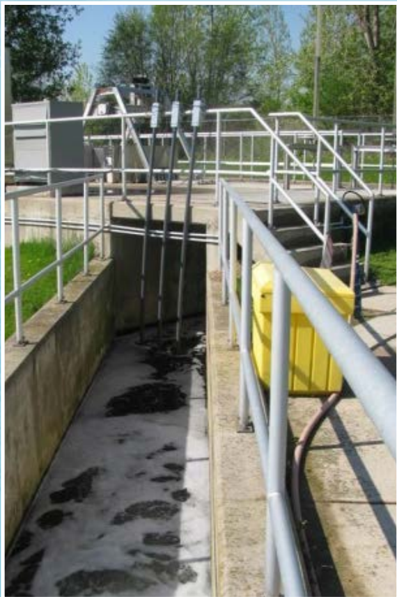
The effluent channel with effluent probes, measuring DO, pH, temperature and TSS
