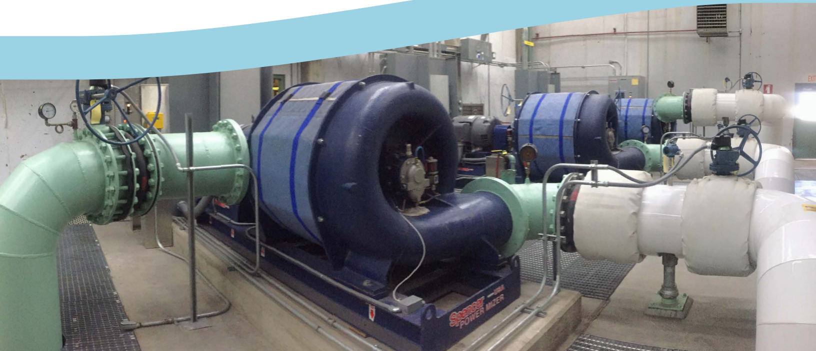
Blowers run more efficiently by monitoring dissolved oxygen
