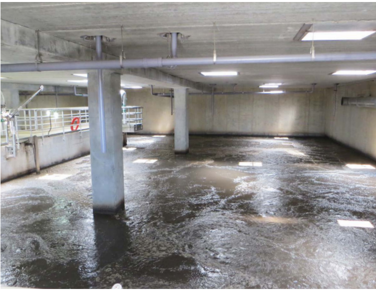
Inside the Douglas L. Smith Middle Basin Plant
