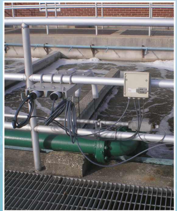
An IQ SensorNet module mounted tank side along with sensors for continuous process monitoring and control.
