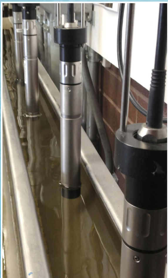
IQSN sensors in effluent
